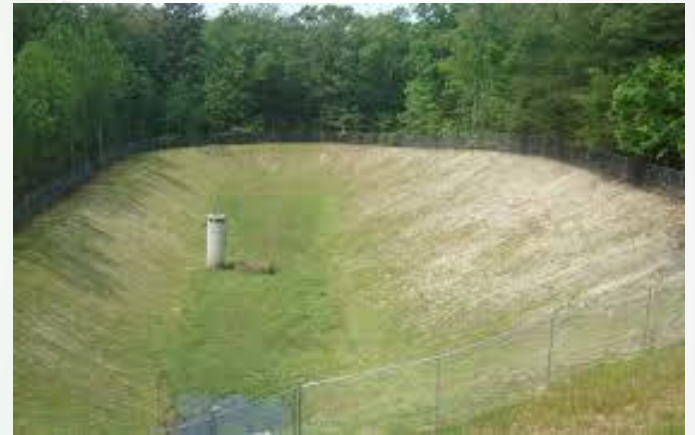
Storm Water Retention Pond
