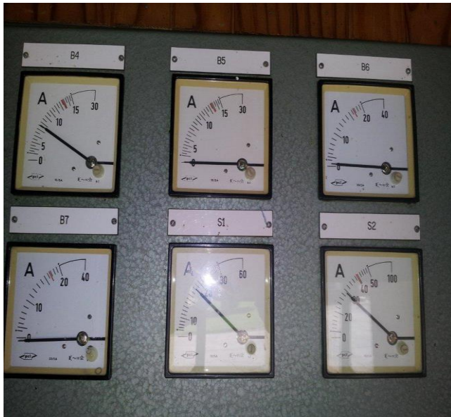
Amp meters which form part of control panel
