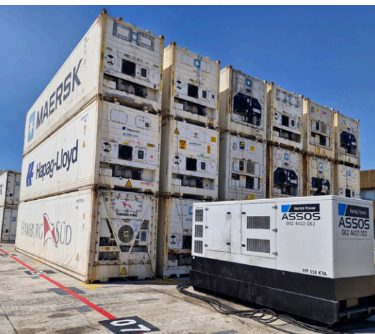
The two 500kVA generators proved effective over three months in preventing container backlogs amid severe weather and power constraints.
