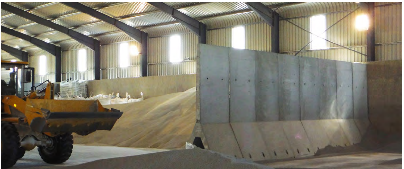
Yfel barriers being used to separate fertiliser products in storage.
